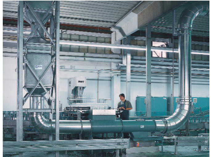
Feed station with supply air plant and conveying duct
